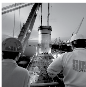
Left: Manifold section of the turret of FPSO Capixaba Right: Lifting operation of the lower section of the Skarv FPSO
