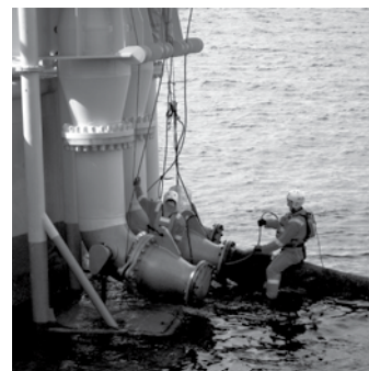
Top: Hook up operation of the marine offloading hose to a deepwater CALM buoy Bottom: SBM Offshore employee
