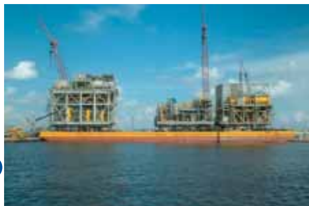
The main modules being offloaded from US yard for transport and installation on board Kuito FPSO as part of phase 2A development.
