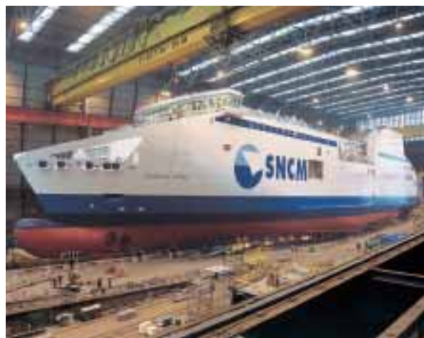
Inside GN's large construction hall the 24-knot Ro-Pax ferry Pascal Paoli for French owners SNCM.
