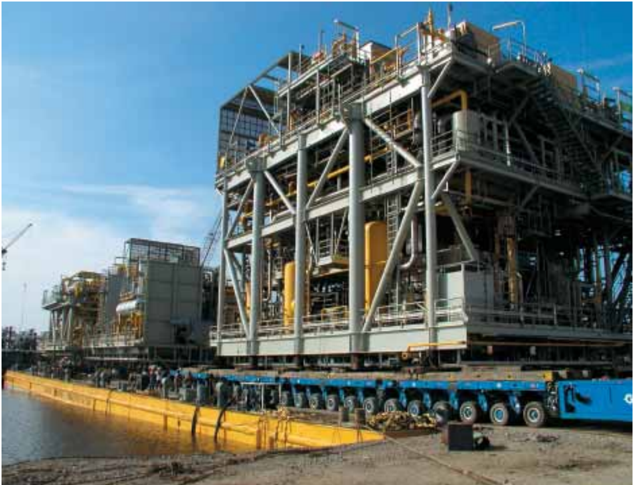
The main modules being offloaded from US yard for transport and installation on board Kuito FPSO as part of phase 2A development.
