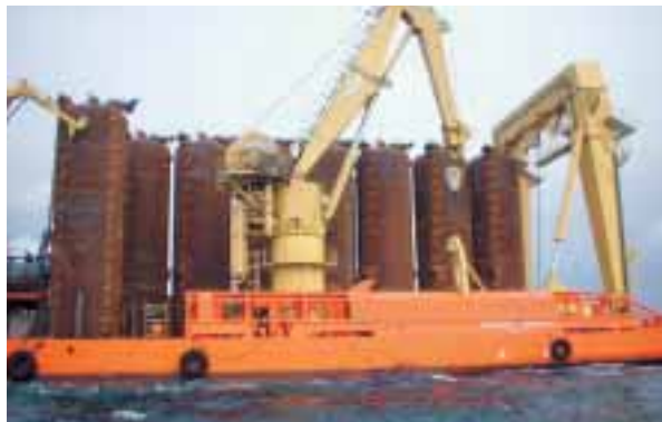
Pre-installation of Serpentina FPSO moorings by SBM's MPV Normand Progress : the nine suction piles ready for launching in 900 metres water depth.
