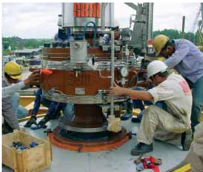
State-of-the-art high pressure toroidal swivel being assembled on the turntable deck
