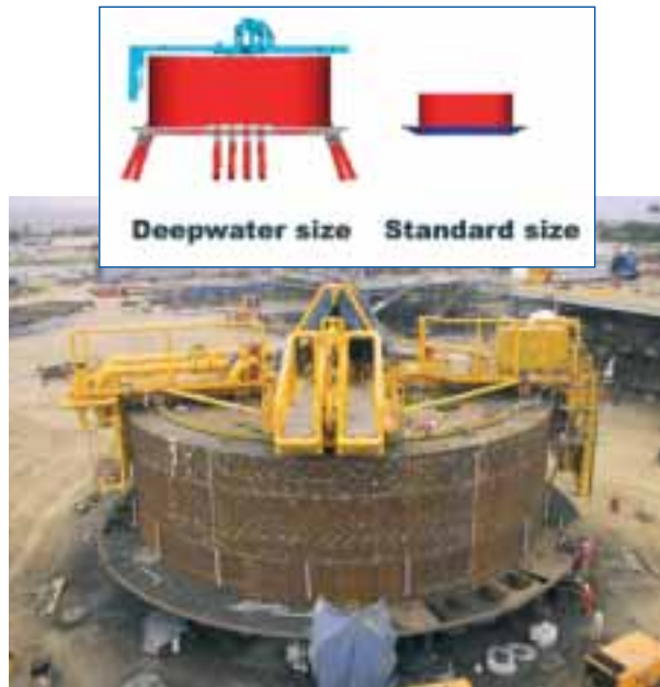
Kizomba A deepwater buoy for block 15, Angola, at final stage of construction in Lobito, Angola
