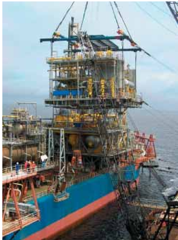
One of the main modules being lifted on board the Kuito FPSO offshore as part of Phase 2 development
