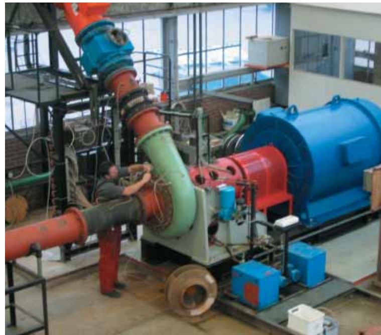
Pump circuit at MTI
