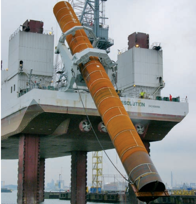
Trials with the pile upending and guidance tool for the installation of mono-pile foundations for wind turbines
