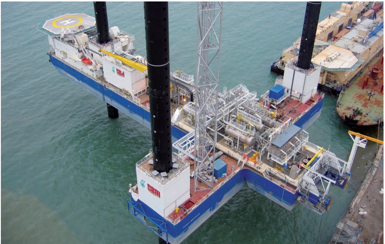
An aerial view of the MOPU for Turkmenistan beside the quay of the assembly yard in Baku
