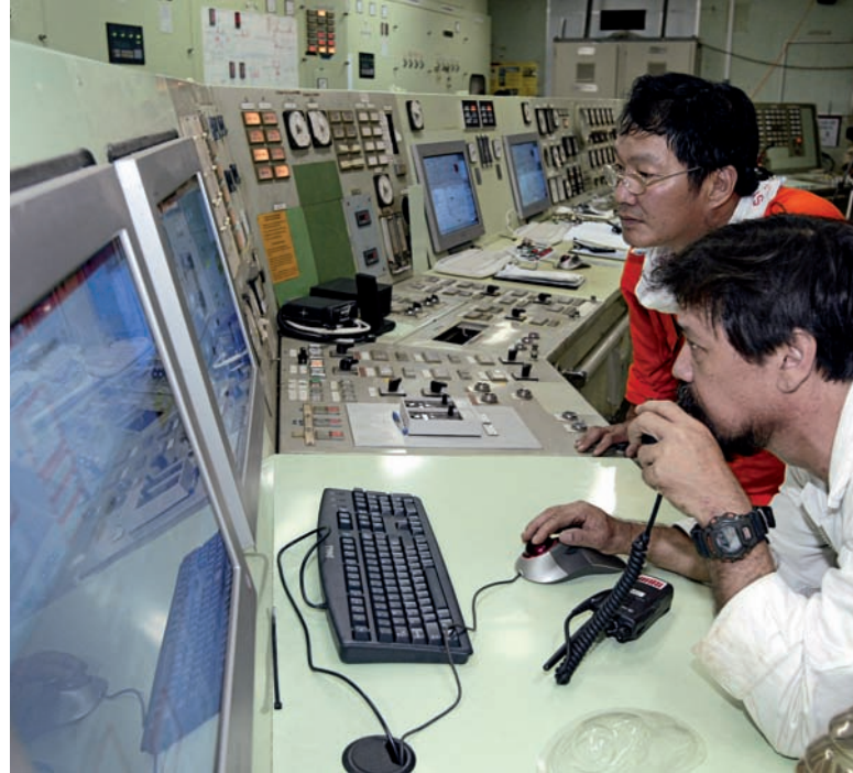
The central control room of the FPSO Marlim Sul offshore Brazil
