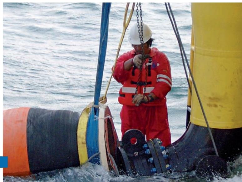
Tie-in of the floating hose string during the installation of a CALM terminal
