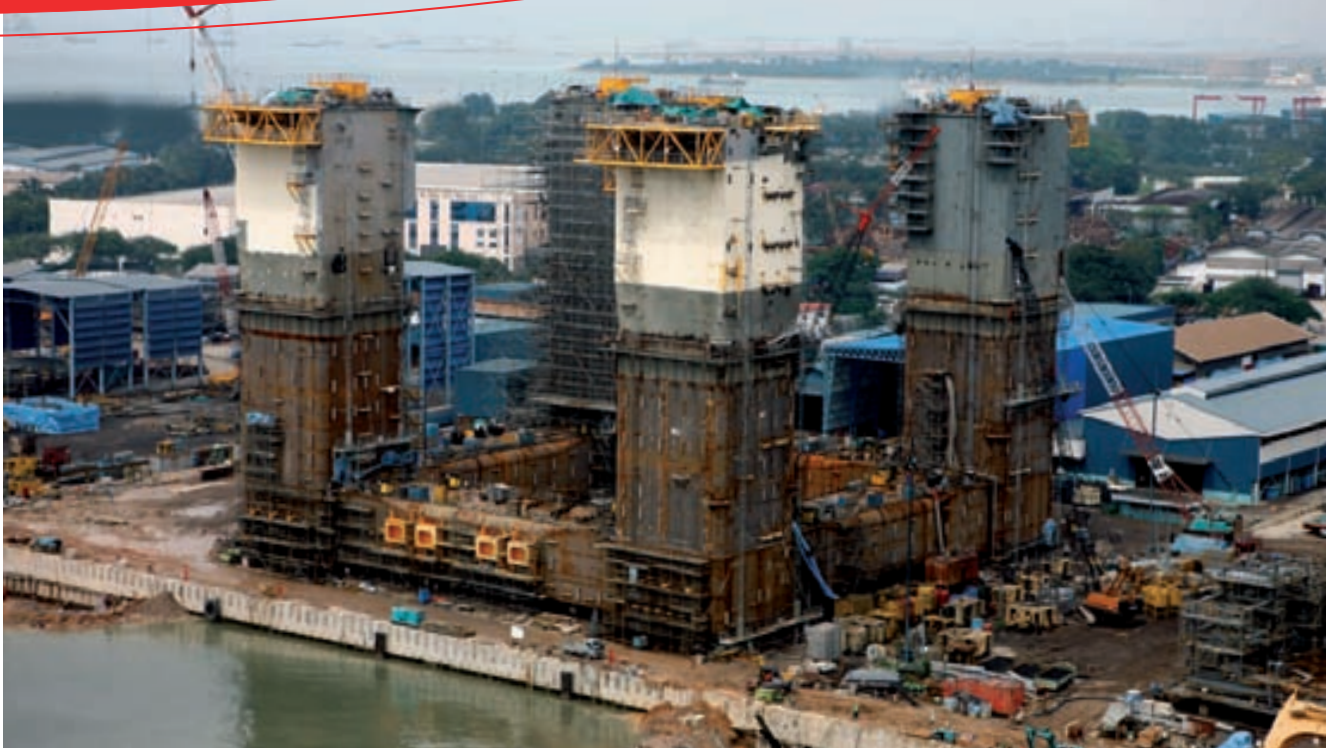
The semi submersible hull for the Thunder Hawk production unit nearing completion in Singapore
