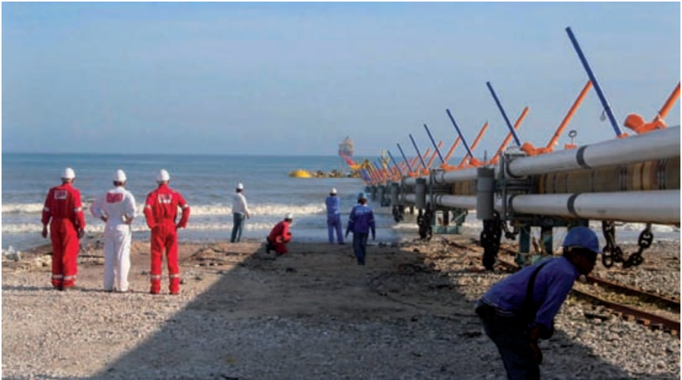
Launching of the GAP™ at the construction site on the coast of Borneo, Malaysia
