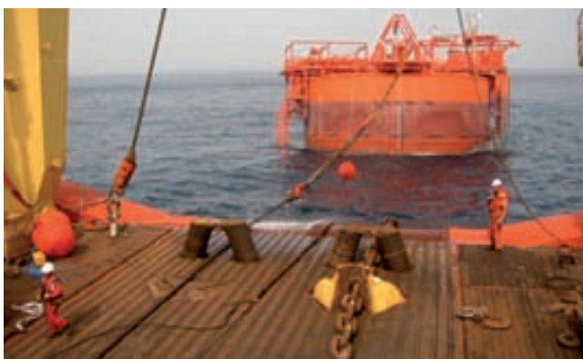
Agbami Deepwater CALM buoy during installation offshore Nigeria with the 'Normand Installer'
