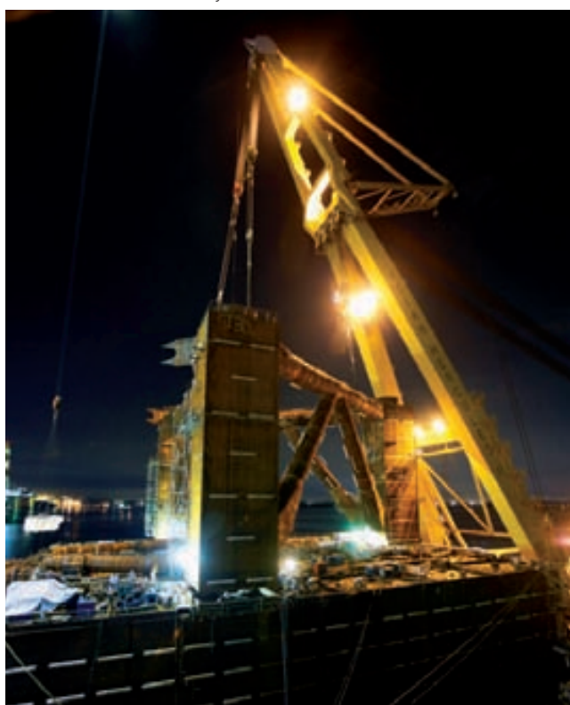
Support structure for the jack up legs being lifted onto the storage tank of the MOPUstor™ in Malaysia
